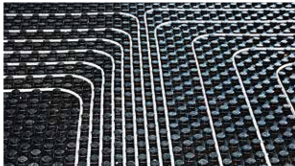
Underfloor heating with nubs
